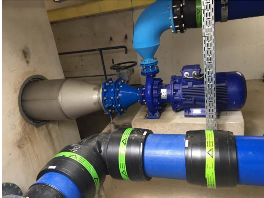
Figure 7: Condition at Surge tank after Installation
